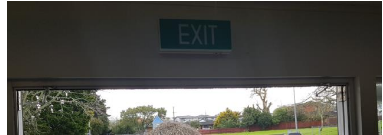
Emergency Exit/Lighting at the Church Foyer (Main Entrance)
